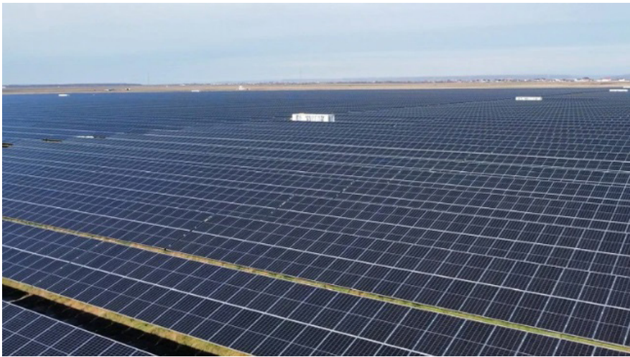
Fig. 12. Photovoltaic park from the southern part of Romania (source: https://earth.google.com ).
